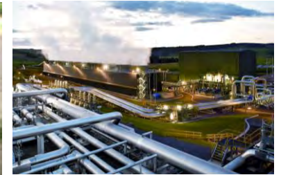
Ngā Awa Pūrua 2 (2010) 138MW 754GWh (Mercury owned 65%)
